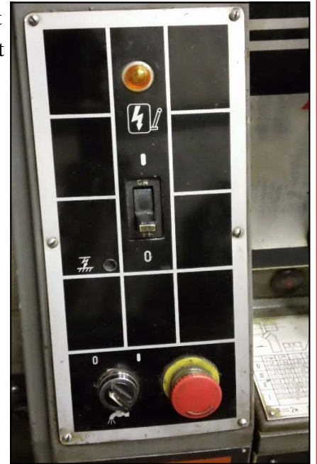
Fig 2A: Control Panel
