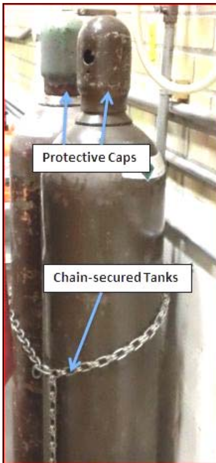
Figure 2O: Tank Storage
